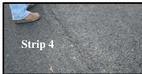
Figure 5.5. Example Mat Tear At Edge of Roller
