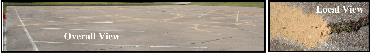
Figure 3.4. Sanded Cracks Prior to Sweeping
