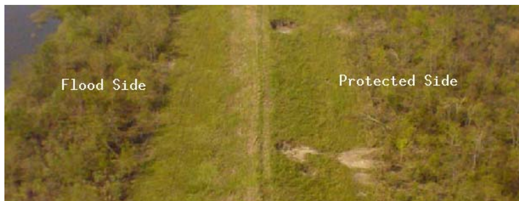
Figure 1.1. Minor erosion due to overtopping on the Citrus Back levee
