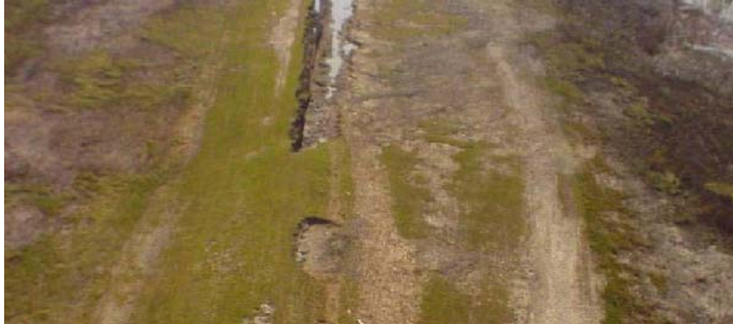
Figure 1.2. Crown erosion along MRGO levee in St. Bernard Parish
