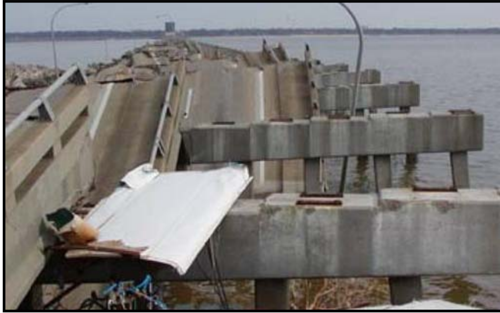
Figure 1.1. Biloxi Bay Bridge-Hurricane Katrina-2005 Atlantic Hurricane Season.
